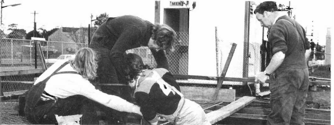
Carpenter Andy Jackson (in white jumper), apprentice Ian Clark (in football jumper), carpenter John Larkins (on right) and labourer Tim Curry (left back ground) at work at Alphington.
