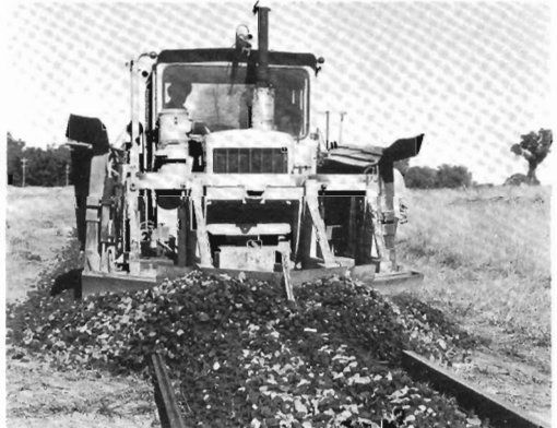
Then the familiar blue metal ballast is spread over the new track.
