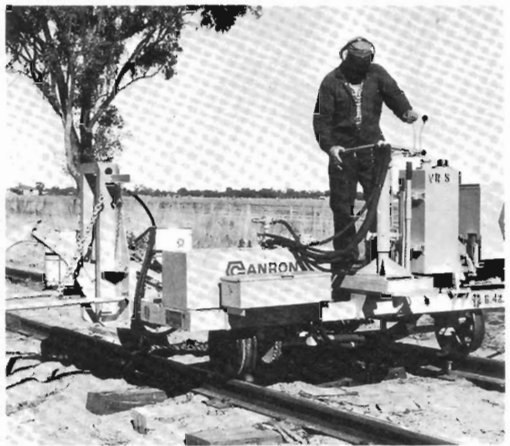
After new sleepers and new rail have been positioned, dog spikes are placed in holes that have already been drilled in the sleeper. Like the dog pullers two dog spikers work on the spikes one working on the inside of the rail and the other on the outside.
